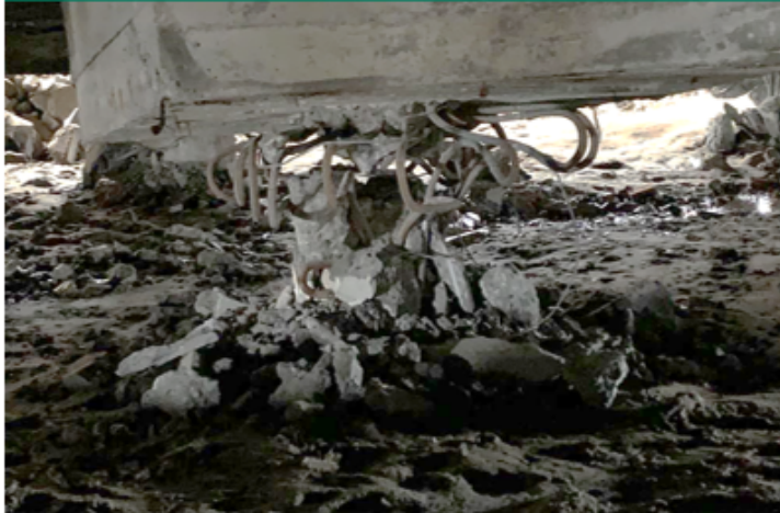
Failure of some of the reinforced concrete piles which supported the tank
