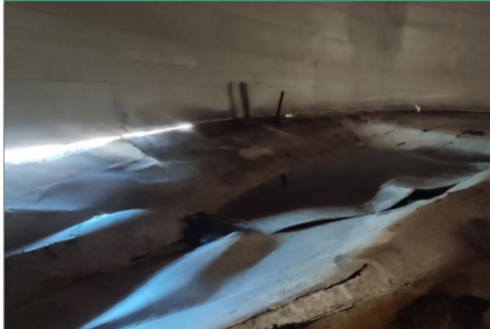
Interior of the tank showing a large depression caused by pile failure which in turn caused failure of the common plates dragging the annulars inwards resulting in failure where the plates met the shell
