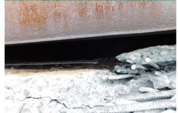
Rupture of the tank shell where the wall is welded to the floor
