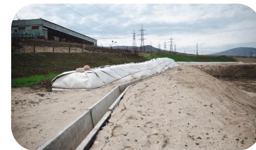
In 2024, a 5.8 ha industrial waste landfill with a capacity of 26.8 ktpa was commissioned in Monchegorsk
